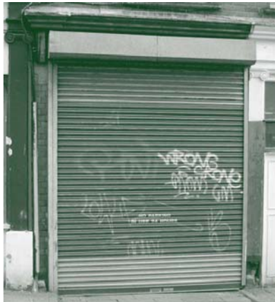
Roller shutters of a solid appearance are unsightly and not generally acceptable.
