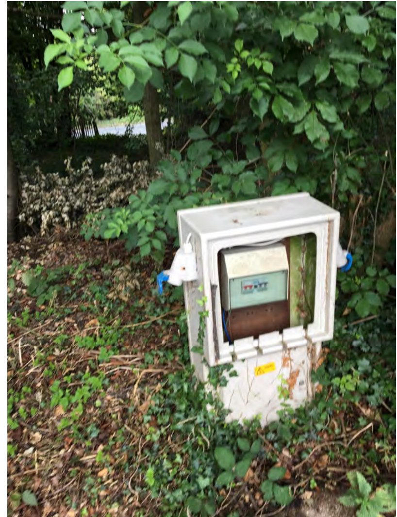
Photo 20: Electricity supplies within caravan site
