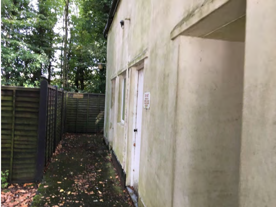
Photo 15: Derelict toilet block in south east of caravan site area
