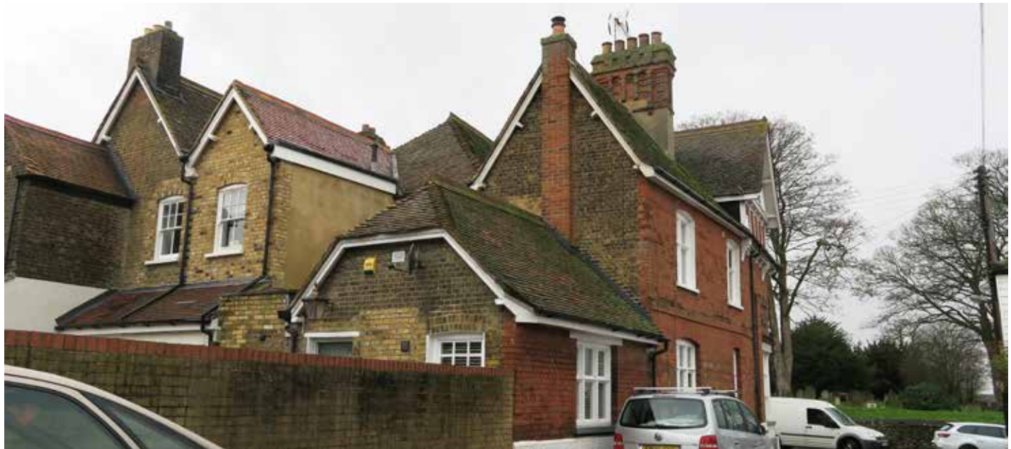
Figure 44: Back of buildings showing a diversity of roof styles, orientations, and pitches.
