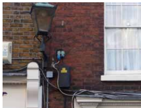
Ad-hoc accumulation of wires
