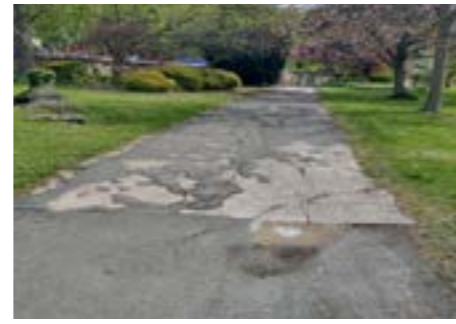
Resurface all paths that are in poor condition
